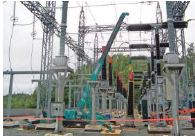
MC405C Power Station Quebec
