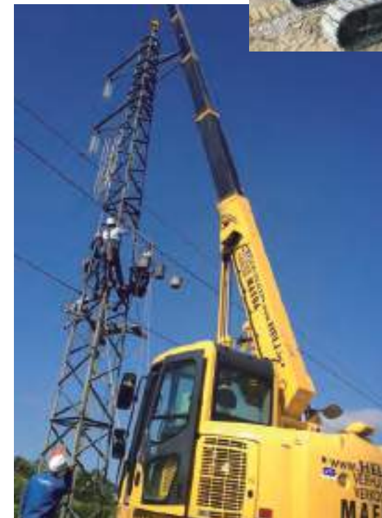
LC1385 Steel Tower
