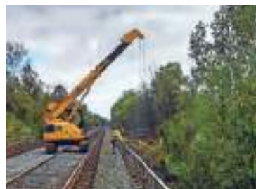
LC785 Railway Difficult Access To Lift
